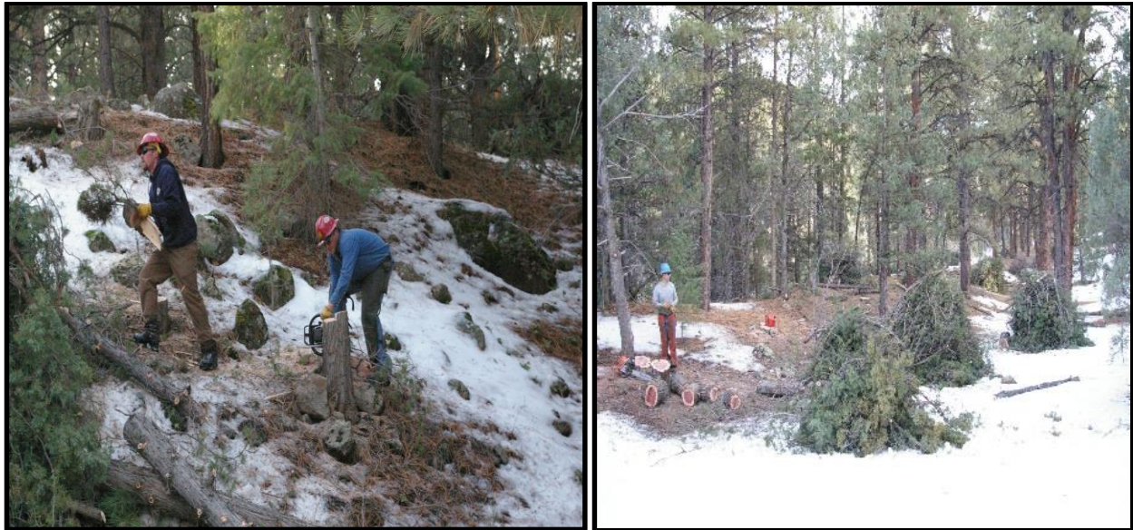
*Photos of Forest Service crews working on the Little Res II project during the Fall of 2015.
